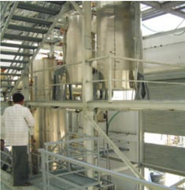
Commercial Plant at Butibori, Nagpur
