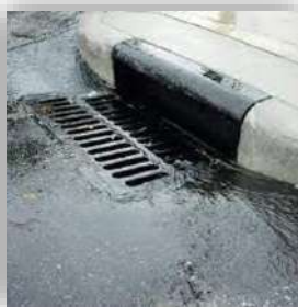
Storm Water Drains
